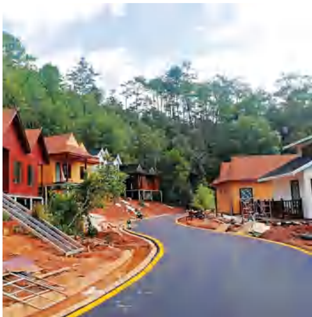
During the pandemic, wooden house construction in APFNet Pu'er SFM Demonstration and Training Base in China. Photo: Li Zhaochen, project manager/APFNet.
